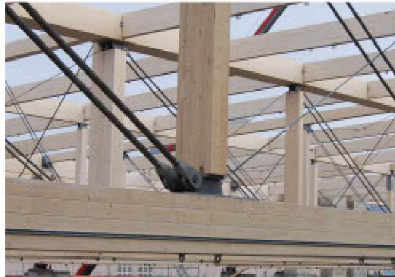
Connection Detail Example- Steel Diagonals introduced to reduce weight WIEHAG Timber Construction GmbH
